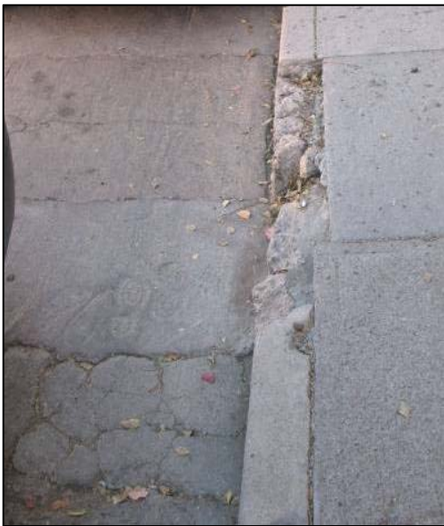
Streets, sidewalks and curbs are patched and crumbling in many areas of downtown.
